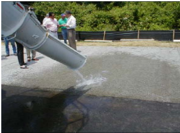
Figure 7. Pervious Concrete at the Girl Scout Program and Learning Center on Lexington Road
